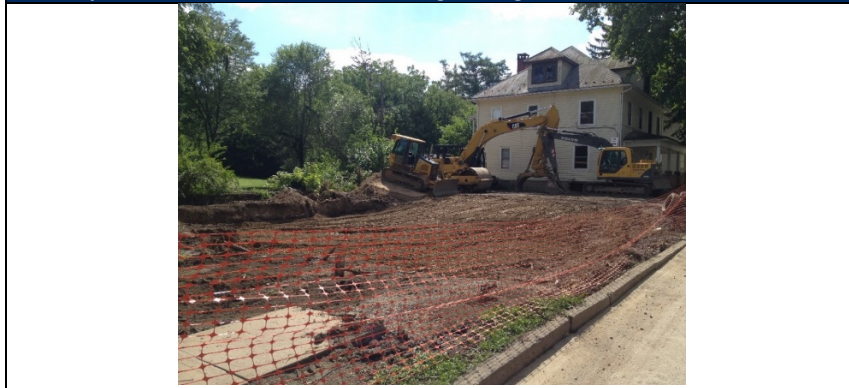
Figure 4.3.3-3 Photo of acquisition and demolition project of several repetitive loss structures in Lewisburg Borough.
